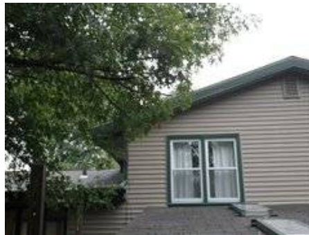
Photo 9-2 Trees overhanging roof lines - recommend trimming back to prevent wood destroying insects damage.
