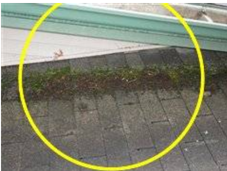
Photo 16-1 Moss growth on roofing shingles - recommend cleaning off to prevent shingle life cycle shortened.
