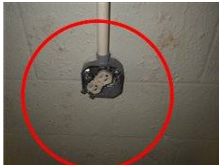
Photo 25-2 Missing cover plate - unsafe condition.
