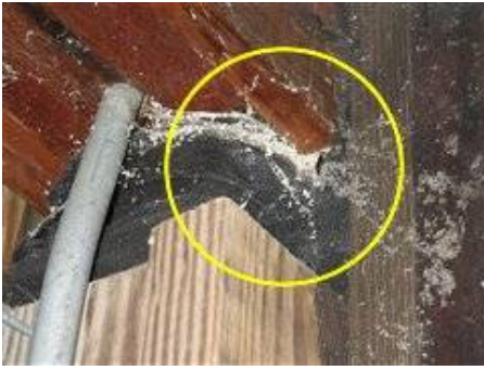
Photo 55-1 Carpenter ant evidence on decorative center beam - recommend treatment for both carpenter bees and carpenter ants.
