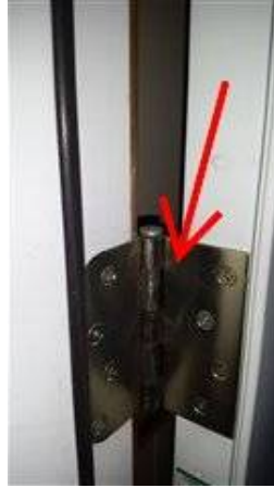
Photo 18-2 Non spring loaded hinge to help aide in metal door fire rating. Recommend adding a spring loaded hinge.
