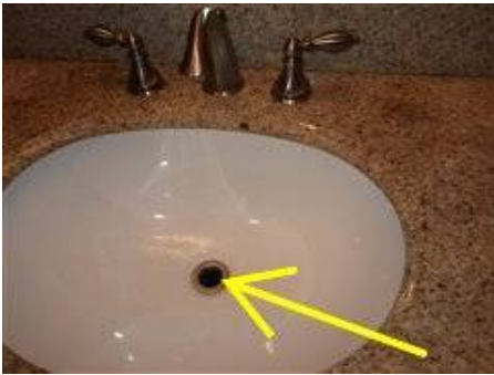
Photo 46-1 Stopper missing in sink
