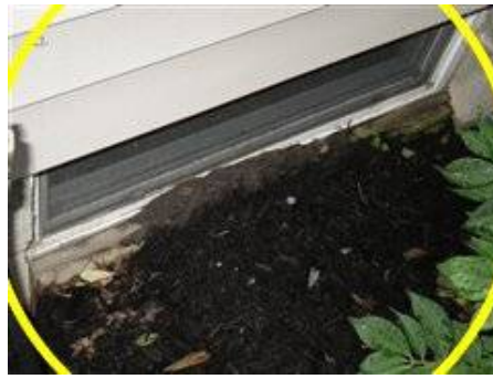
Photo 7-2 Soil and mulch against window ledge and wood framing. Recommend keeping soil min. 6" away.
