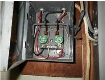
Photo 20-1 Two 30amp fuses for dryer service. Recommend replace to a breaker sub panel or replacing main panel with an upgraded 150 amp service panel to eliminate.
