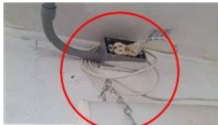
Photo 25-8 Cover plate missing in garage. Safety hazard
