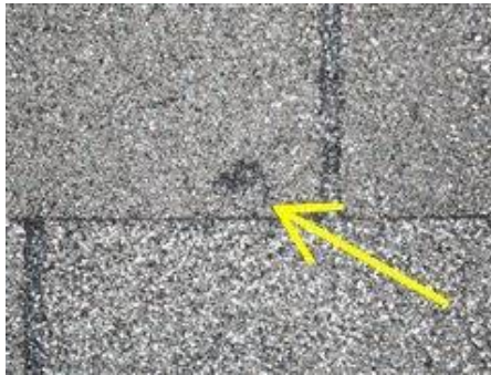
Photo 15-4 #4 Missing granules on a few shingle tabs - monitor or seal.
