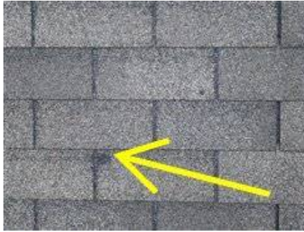
Photo 15-2 #2 Missing granules on a few shingle tabs - monitor or seal.
