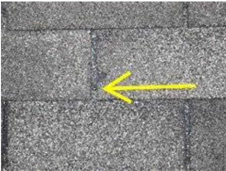
Photo 15-3 #3 Missing granules on a few shingle tabs - monitor or seal.
