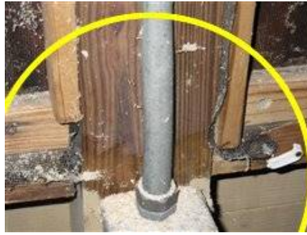
Photo 55-2 Wood destroying insect damage evidence.
