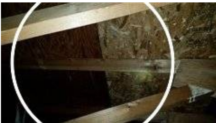
Photo X-3 Previous repaired roof sheeting
