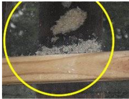
Photo 56-2 Evidence of carpenter bee damage. Recommend plugging holes with a butyl caulk to prevent reuse next season.
