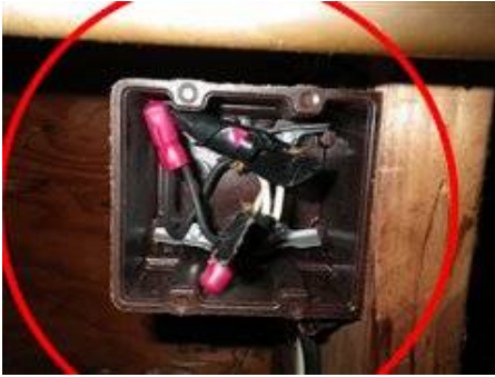
Photo 25-5 Cover plate is missing.
