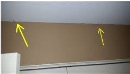
Photo X-1 Nails popped - remove and patch
