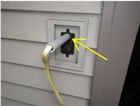
Photo 8-1 Gap around plastic conduit needs sealed or caulked.
