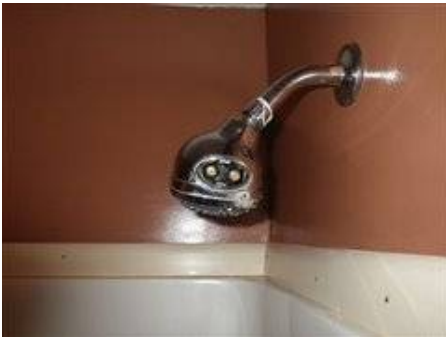
Photo 48-1 Shower head missing cover plate.
