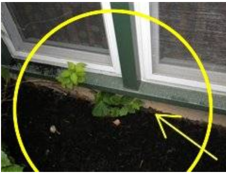
Photo 7-1 Soil and mulch against wood framing under window. Recommended to be min. 6" below.
