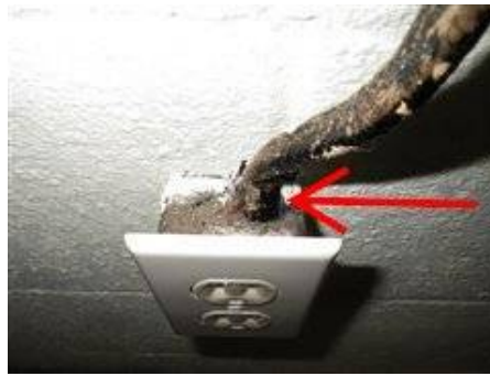
Photo 22-4 Improper connection as wire connector is not used and wire is loosely hanging on wall. Unsafe condition
