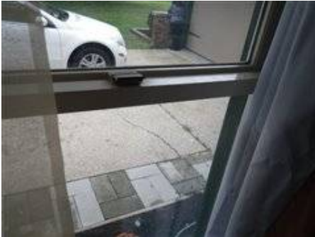
Photo 50-1 Craftline Double hung window was stuck and did not open when tried.
