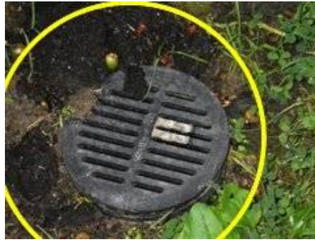
Photo 5-2 Drain grate is set to high to soil around - grading and sloping away from foundation is need all along north end of house to prevent water intrusion.
