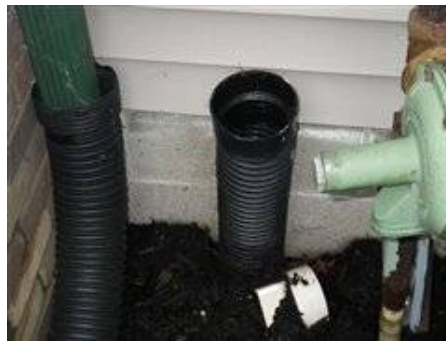
Photo 5-4 Open drain without grate cover but unable to tell need or use for it? Could clogged other lines if not capped.
