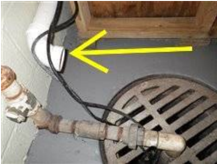
Photo 47-1 Washer drain piping needs extended down to sump crock to prevent water collecting on floor around sump crock.
