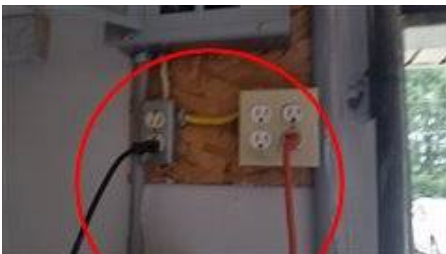
Photo 22-7 Outlets in garage are non GFCI outlets as now recommended.
