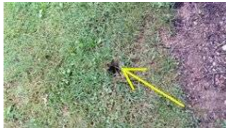
Photo 5-6 Open drain without grate cover. evaluate drain system and need.
