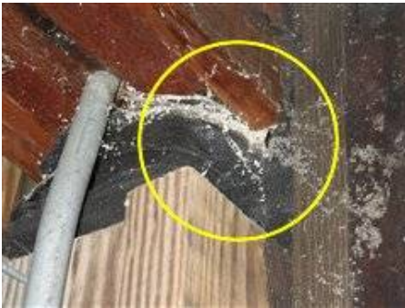
Photo 55-1 Carpenter ant evidence on decorative center beam - recommend treatment for both carpenter bees and carpenter ants.
