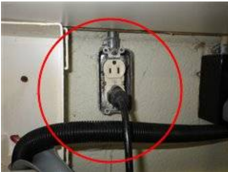
Photo 25-1 Missing cover plate - unsafe condition.
