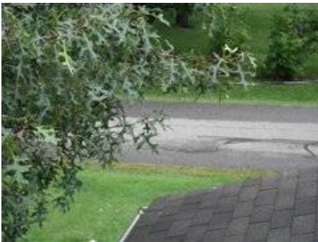
Photo 9-1 Trees overhanging roof -recommend a tree arborist trim back off roof line to prevent wood destroying insects.
