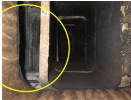
Photo 41-2 Clay flue liner in chimney is offset and needs evaluated by a qualified masonry contractor with chimney repair work.
