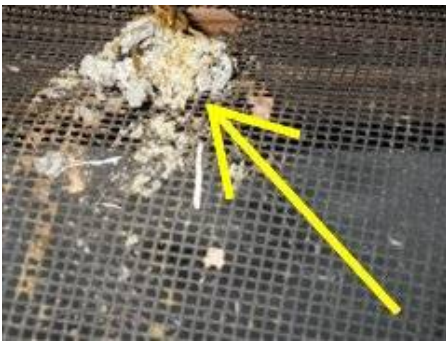
Photo 56-1 Evidence of wood destroying Carpenter bees on patio privacy wall/screening.
