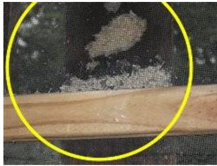
Photo 56-2 Evidence of carpenter bee damage. Recommend plugging holes with a butyl caulk to prevent reuse next season.
