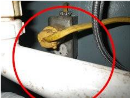
Photo 22-5 Food disposal outlet is a non GFCI outlet as recommended. Have a licensed electrician repair all electrical issues.
