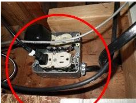
Photo 25-7 More unsafe conditions from missing plate covers
