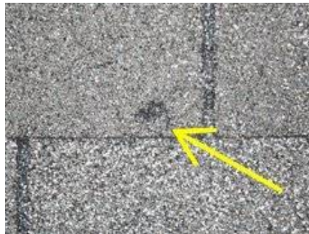
Photo 15-4 #4 Missing granules on a few shingle tabs - monitor or seal.
