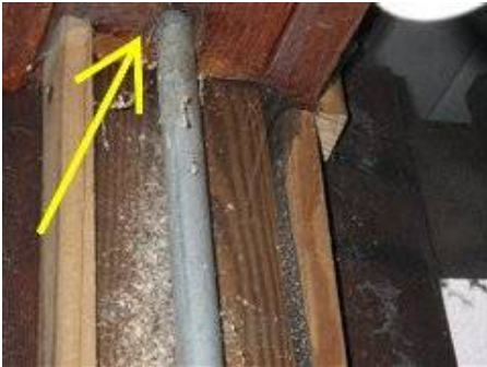
Photo 56-3 Wood destroying insect damage evidence.
