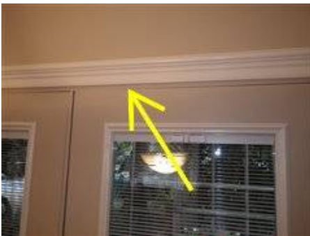
Photo 51-1 Double door needs re-aligned. Recommend trying adjust with 2 1/2" to 3
