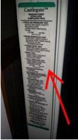
Photo 18-1 Non-fire rated garage - house entrance door.
