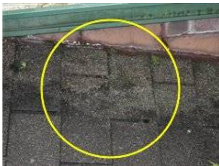
Photo 16-2 Moss growth on roofing shingles.
