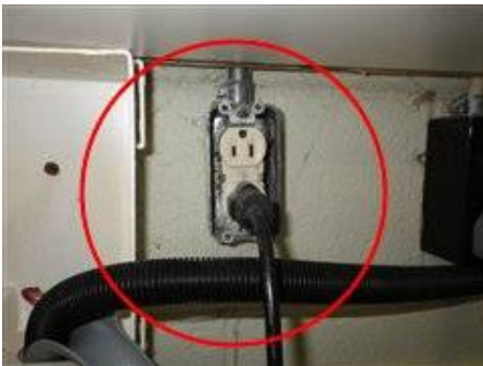
Photo 25-1 Missing cover plate - unsafe condition.
