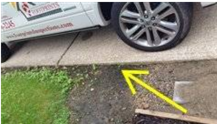
Photo 5-5 Grading along driveway being washed away due to downspouts empty against. This will erode soil under and allow shoving and heaving which will damage concrete driveway. Relocation of downspout needs done soon.
