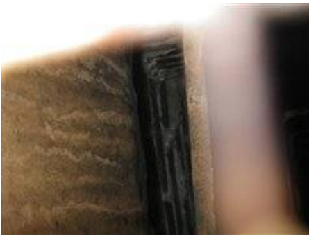
Photo 41-1 Clay flue liner in chimney is offset and needs evaluated by a qualified masonry contractor with chimney repair work.
