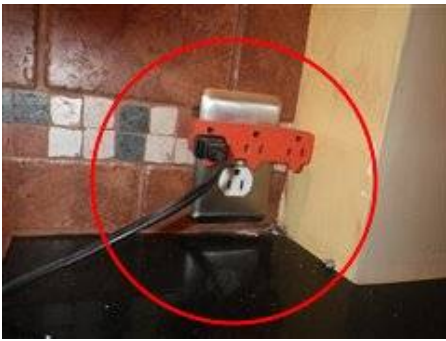
Photo 22-3 Outlet by sink needs to be replaced with a GFCI outlet.
