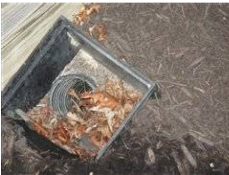
Photo 5-3 Missing grate cover and is sitting to high.
