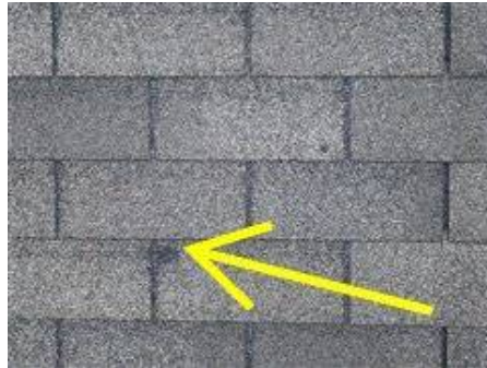
Photo 15-2 #2 Missing granules on a few shingle tabs - monitor or seal.
