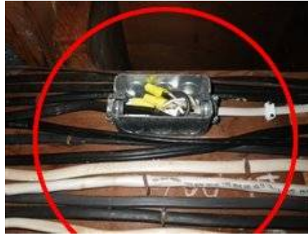
Photo 25-6 Cover plate is missing.
