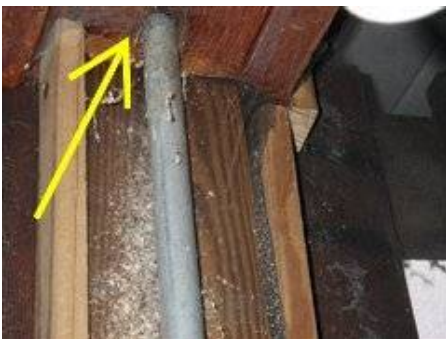
Photo 56-3 Wood destroying insect damage evidence.
