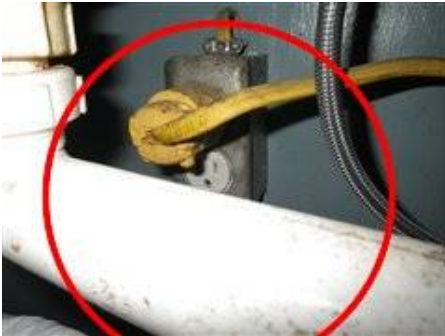
Photo 22-5 Food disposal outlet is a non GFCI outlet as recommended. Have a licensed electrician repair all electrical issues.
