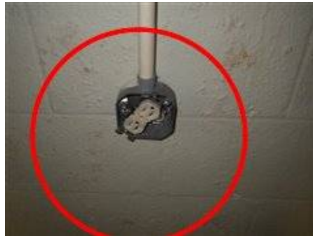
Photo 25-2 Missing cover plate - unsafe condition.
