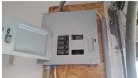
Photo 22-6 Additional service panel with breakers in garage.
