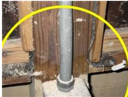
Photo 55-2 Wood destroying insect damage evidence.
