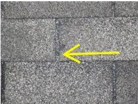
Photo 15-3 #3 Missing granules on a few shingle tabs - monitor or seal.
