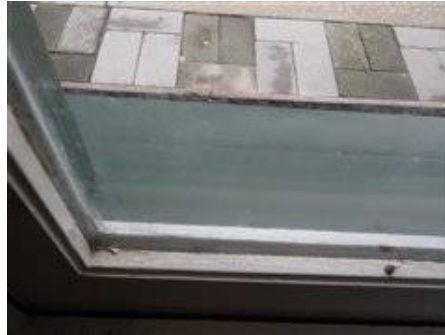
Photo 50-2 Stuck window frame.
